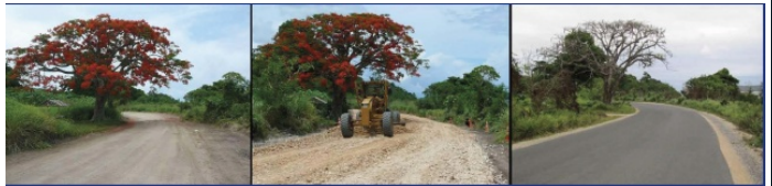
A segment of the Efate ring road, before, during, and after the project.
